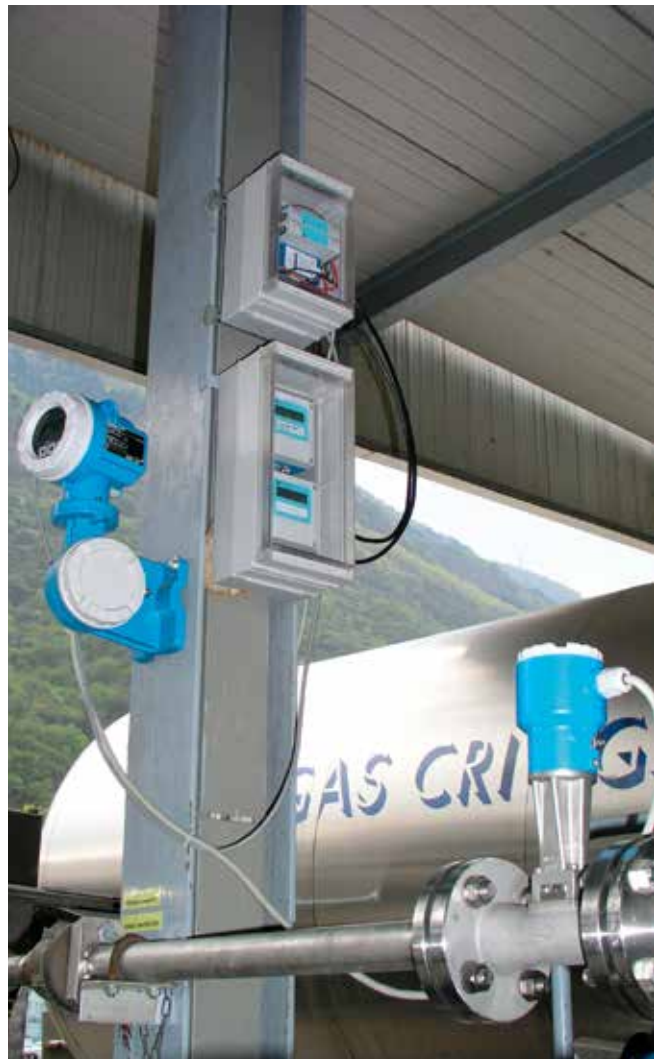
2 Minilog B devices for level measurement and dosing.
