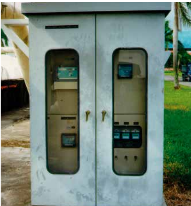
4 Minilog B devices record wastewater inflow on a large treatment plant in South East Asia.
