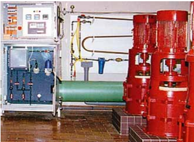
Automatic pump operating time recording using the Minilog B.
