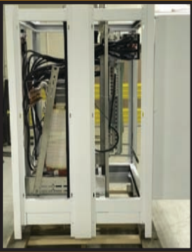
Isolation Transformer & Panelboard
