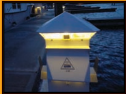
Protected KWH Counter
