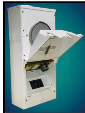
Receptacles and breakers under lockable, weatherproof door
