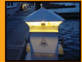
Protected kWh Counter
