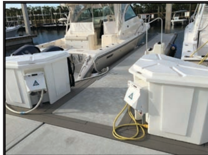
Bayside Mounted in Dock Box
